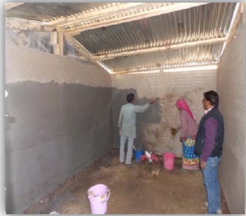
Jute insulation inside a temporary shelter
